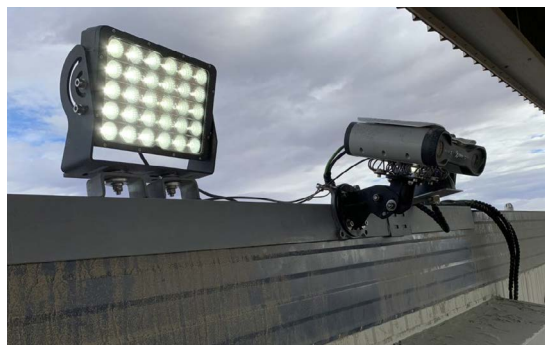
FRAGTrack™ Crusher installation
