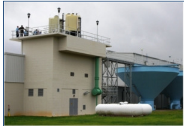
Johnston County water treatment plant in North Carolina, United States of America, the largest MIEX ® system in operation.
