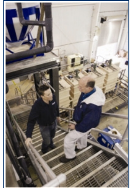
Scott Mitchell, Orica Watercare project manager, working onsite at Arab water treatment plant.
