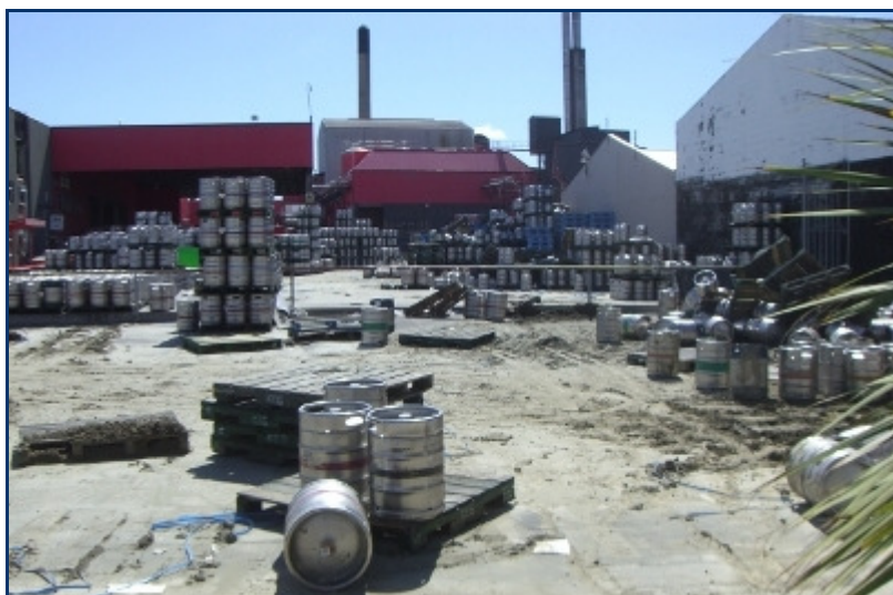
At the Lion Brewery, the soil underneath the thick concrete slab in the yard emerged during the earthquake. Quick action by the Orica team enabled the site to restart production.
