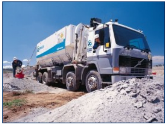
Orica Mining Services delivers ONYX based ANE explosives into blastholes during trials in the Hunter Valley.
