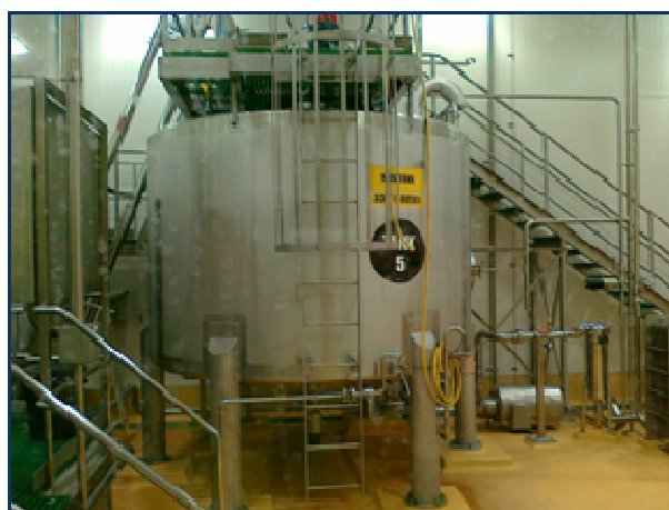
The tank at food grade plant where CIP washings will be used when making subsequent batches of product.
