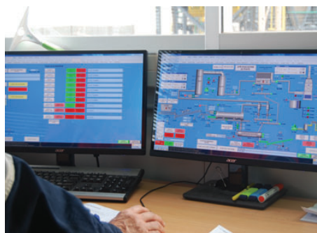
Operating information for the DTD Plant can be closely monitored.
